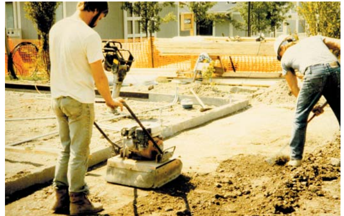
Fig. 1.2 Compaction is necessary to create a load-bearing surface on which to lay pavement.
